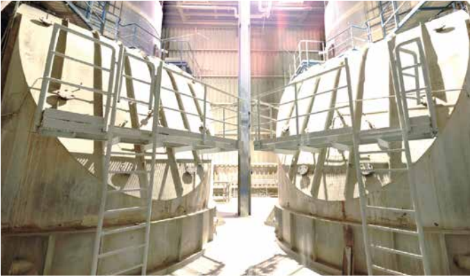
Photo of the plant
